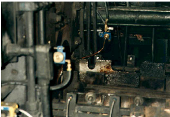
Figure 4: Remote mounting of nozzles away from the heat allows for easy adjustment and repair.
